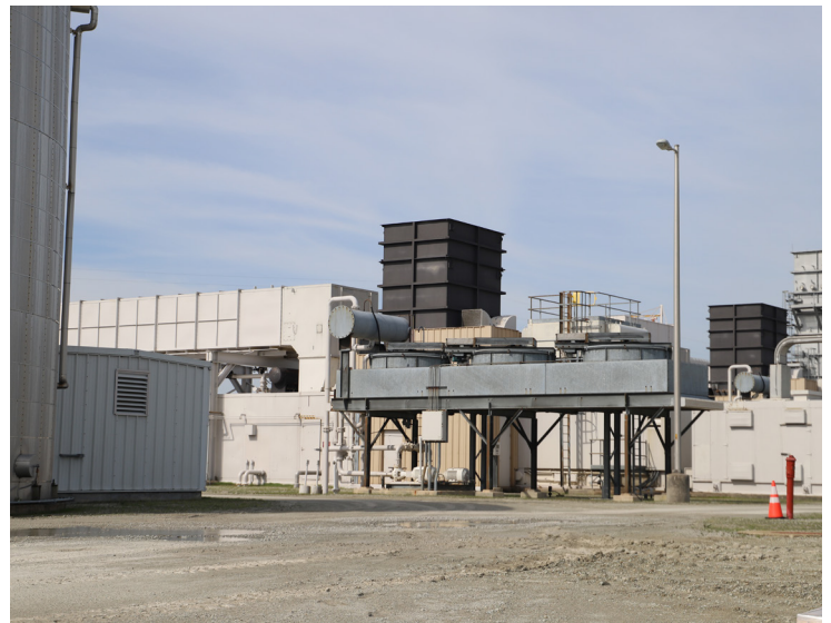
IMPA's Combustion Turbine facility in Anderson, Indiana.
